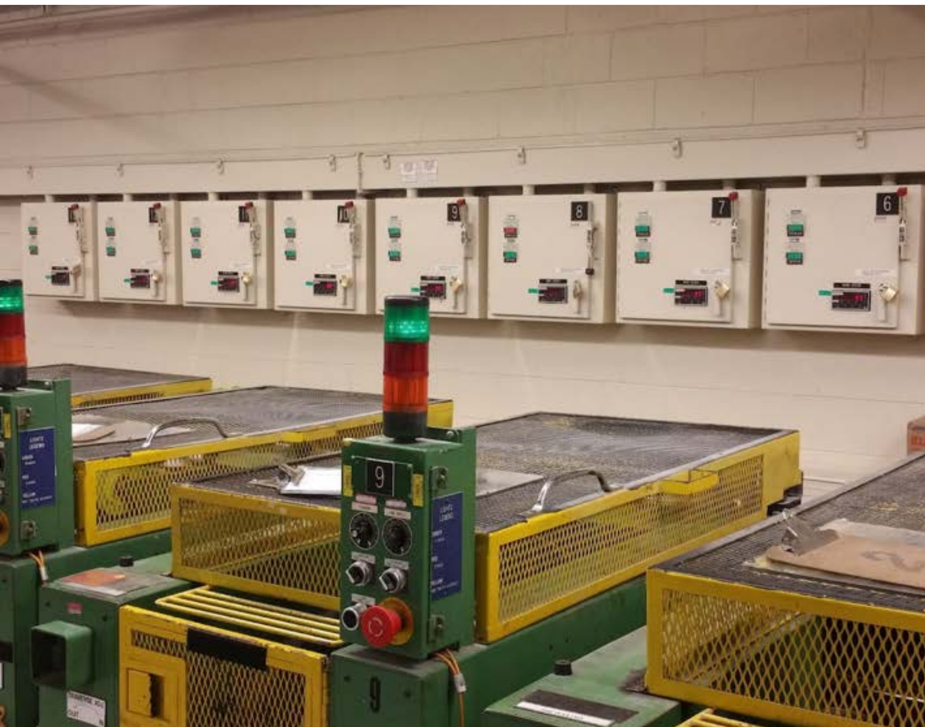
BEFORE: DC DRIVES MOUNTED ON WALL
